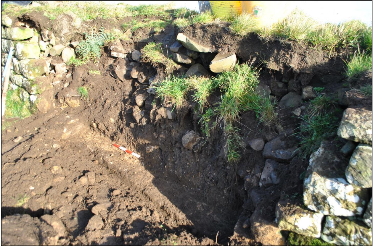
Fig 2: the sound course of probably undisturbed foundation stones with mortar visible, looking north-west
