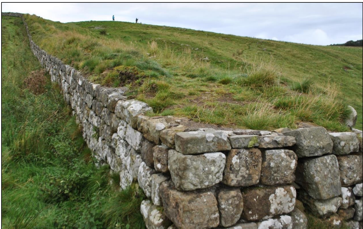
Fig. 2: signs of erosion on the wall top on the northern side of the field gate into Peel Bothy field, looking north, October 2020.
