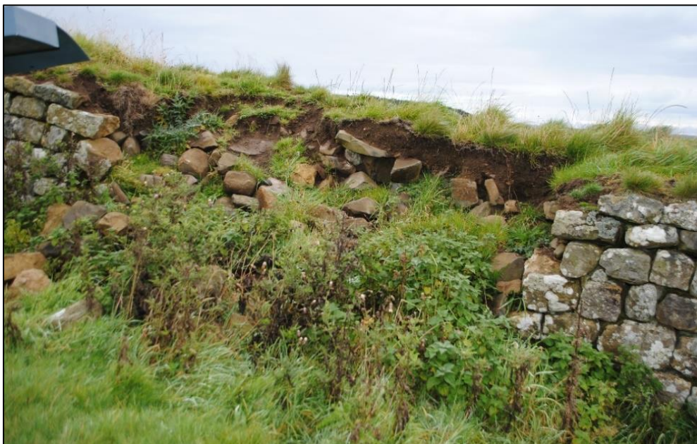
Fig. 6: the failed section in Peel Gap, west slope, October 2020 looking north
