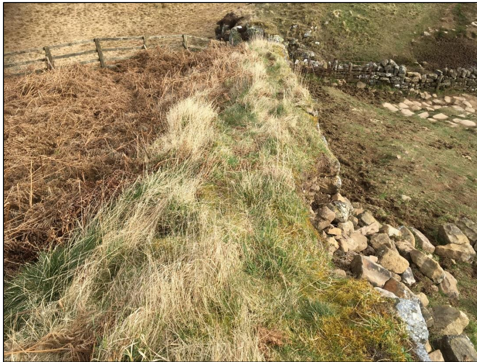
The failed section facing east
