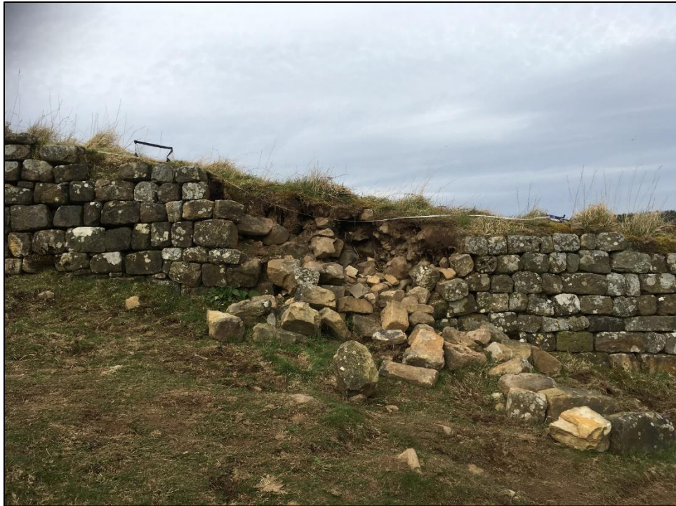
The failed section facing north
