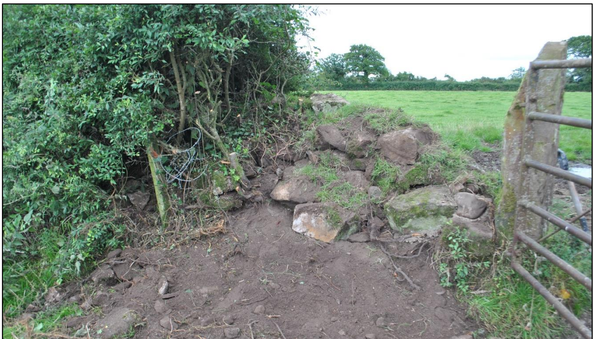
Fig. 1: east of the old gate showing the north 'face' after removal of the hedge (as to left) and initial tidying and turf capping. All the core material was loose and had been re-piled in the past. South-east facing photo
