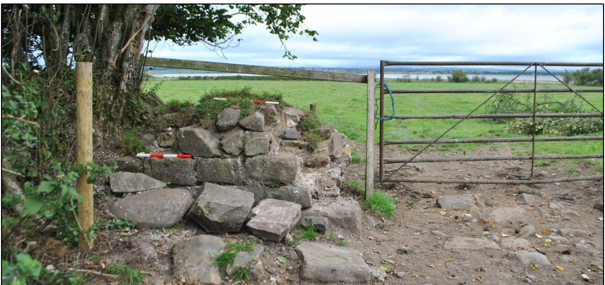
Fig. 5: consolidated Wall west of the gateway before the final re-fencing. Photo looking north-north-east.
