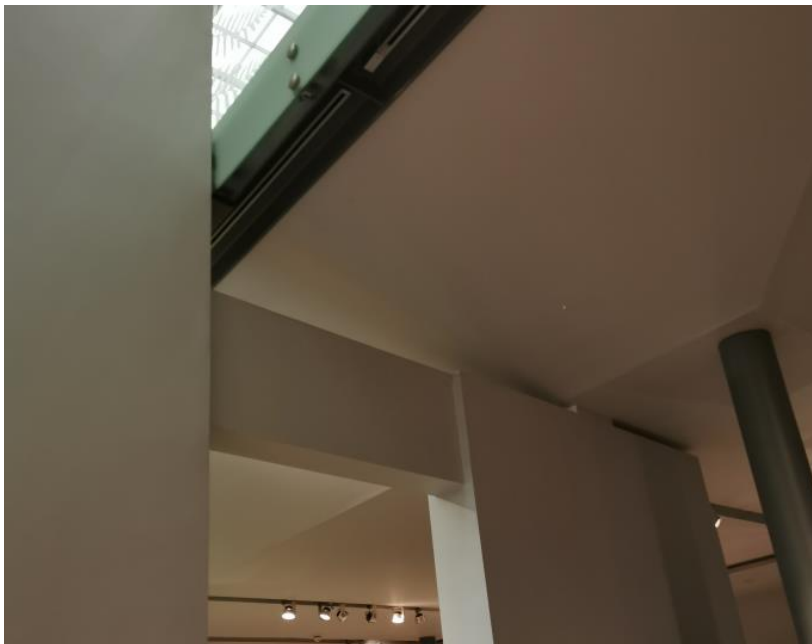
Figure 5: The ceiling above and in front of area 2.
